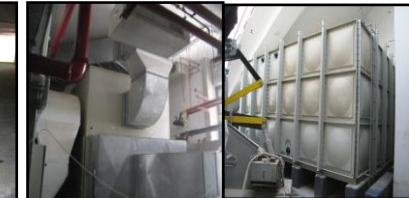
MEP progress at the technical floors showing the final installation of the FAHU & the water tanks
