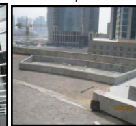
5th floor water feature
