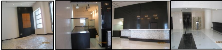
5 th Floor Meeting Room Progress of Works on Ground Floor Reception Hall & Cafeteria
